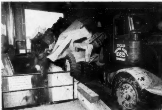
SIDE DUMP TRUCKS are used for long hauls so no time is lost in backing to crusher to dump 400 loads per day.
